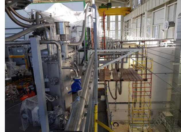
Strings for cryogenic pipes and cables hold
